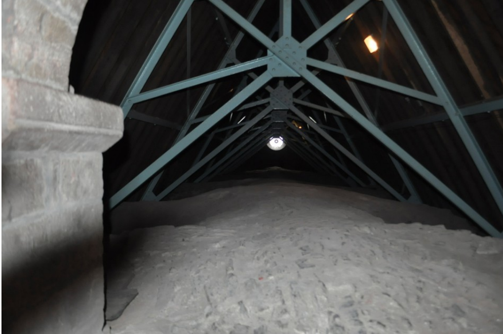
St Magnus Cathedral showing the partial earth brim used to support the ceiling construction.
